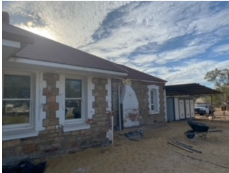
View looking northeast showing part of the east wall of the Darkan Hotel after the demolition of the previous patios.
