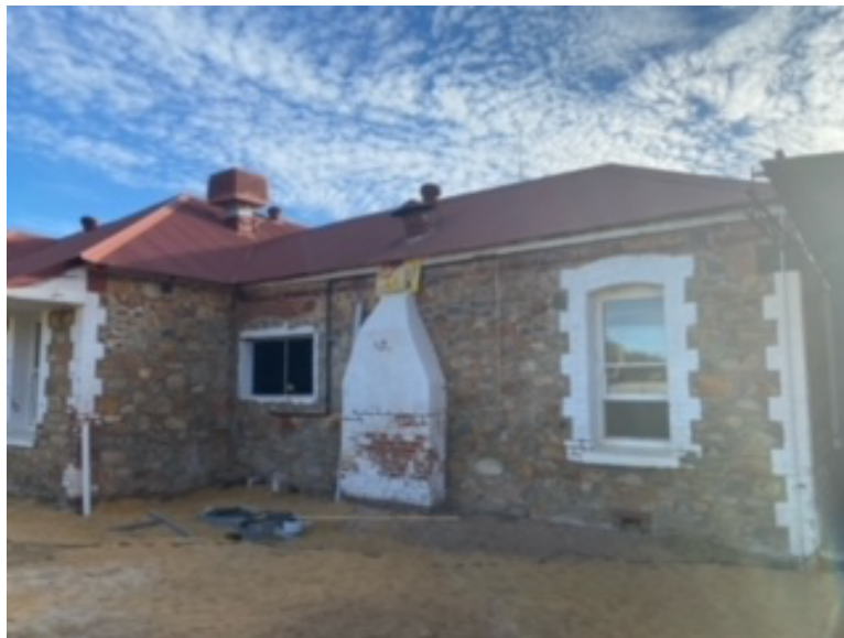
View looking southeast showing part of the east wall of the Darkan Hotel after the demolition of the previous patios.
