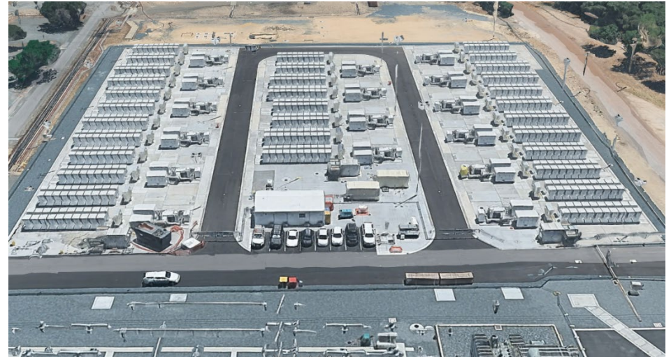
Figure 12: Example of a Battery Energy Storage System
