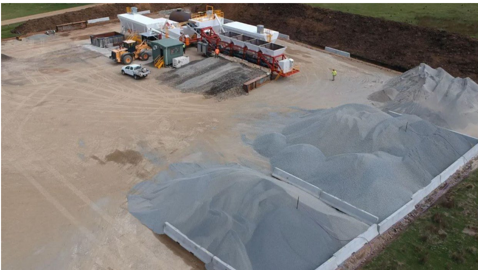
Figure 22: Example of Concrete Batching Plant
